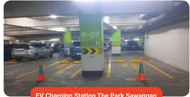
EV Charging Station The Park Sawangan
